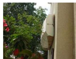
Sliding down the wall!
